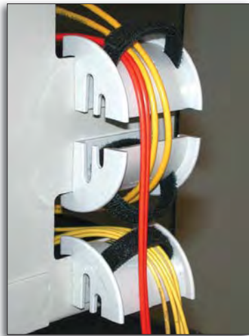
Patch Panel Egress
